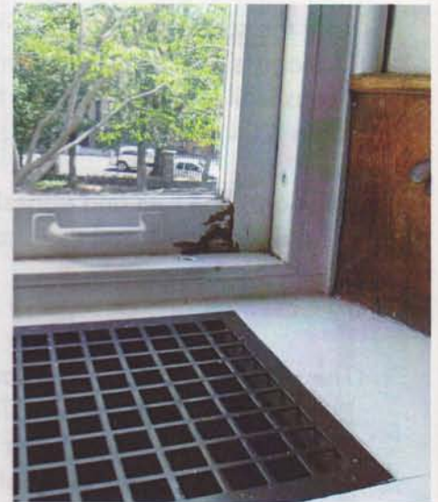
Water damage at Meeting Room (201) windows
