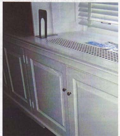
Air handling unit inside cabinetry at the Library/Parlor
