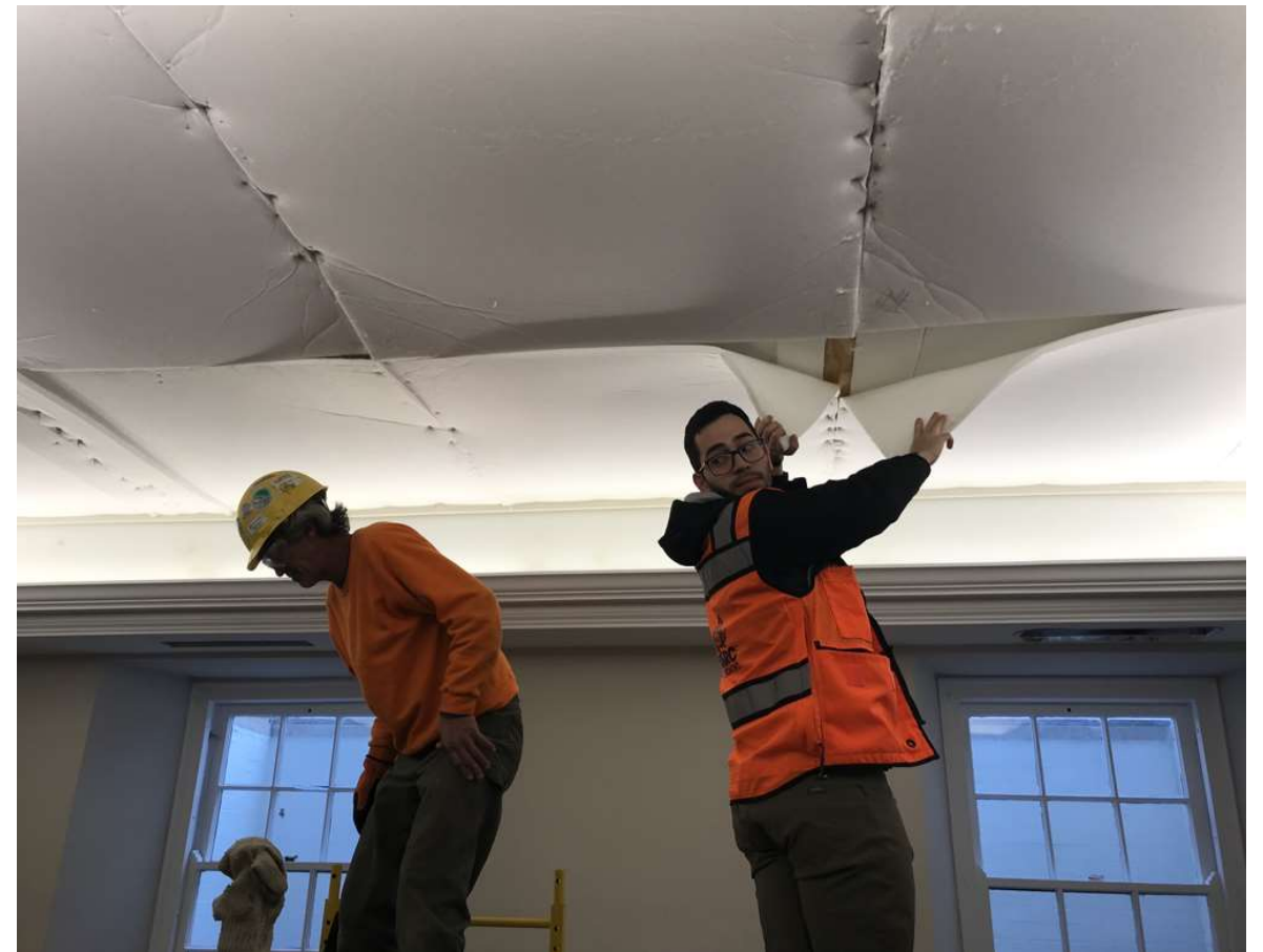
The ceiling installers add in the missing acoustic insulation, here pointed out by Monarc Assistant Project Manager Daniel Berrios.
