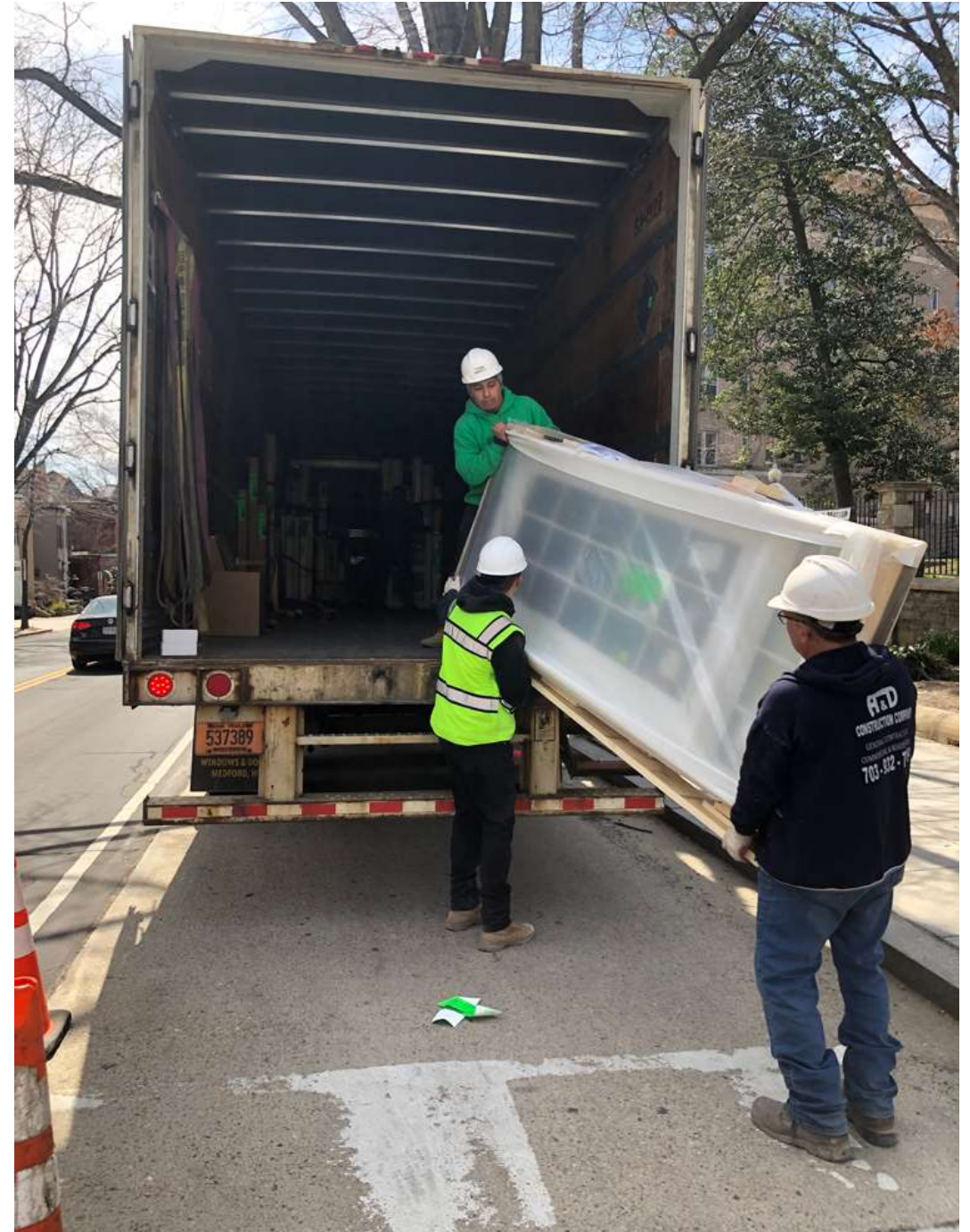
And some Assembly Room doors.
