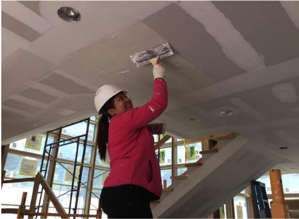
Eight carpenters work on a closet, Lobby windows, architectural metal, and of course drywall.
