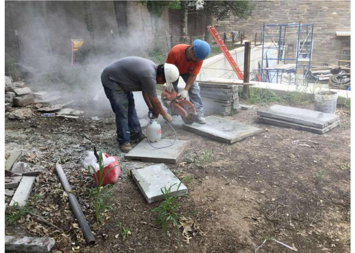
A pair of masons cut up bluestone into risers for the front steps.
