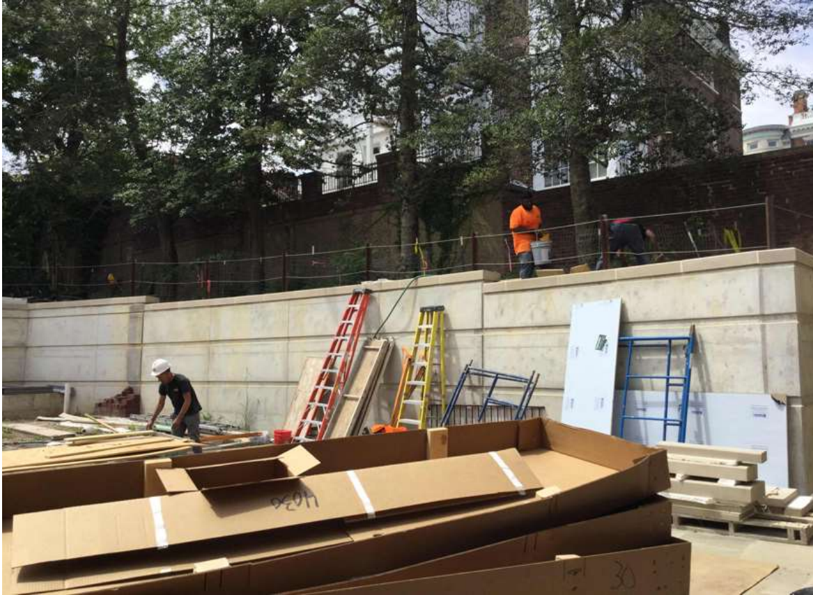
Tyrone and Tyrone nearly finish the cable rail post holes above the retaining wall.
