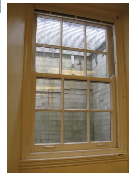
Areaways around basement windows where drains are becoming clogged
