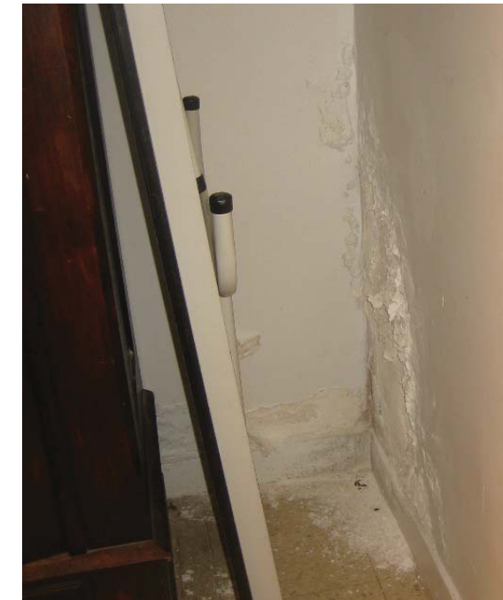
Water damage in Decatur Room
