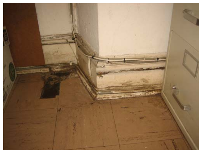
Baseboard at office (108)
