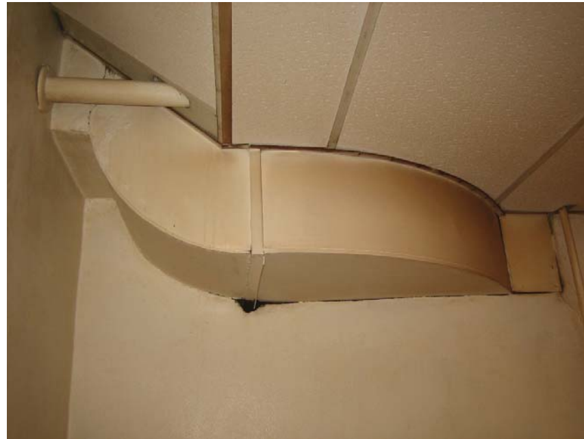
Ducts in kitchen coming from furnace room
