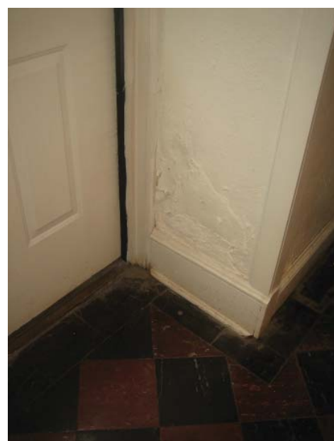
Water damage at west kitchen wall
