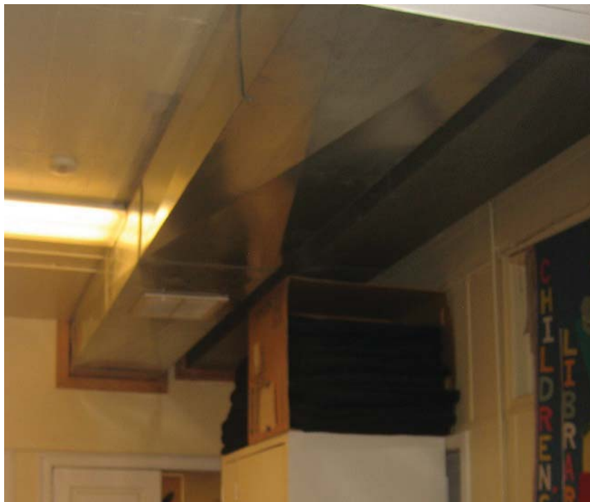
Ducts in hallway (105)
