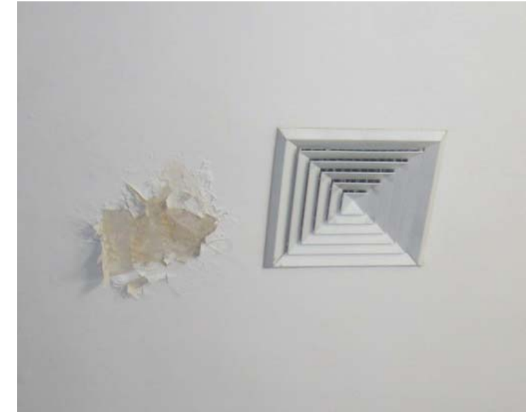
Damaged plaster ceiling in Meeting Room (201) from a roof leak
