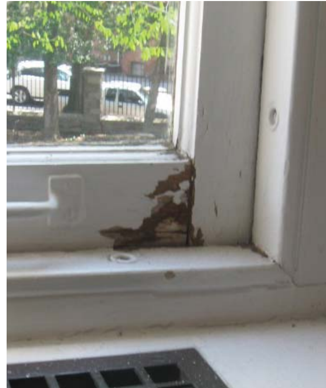
Water damage at Meeting Room (201) windows
