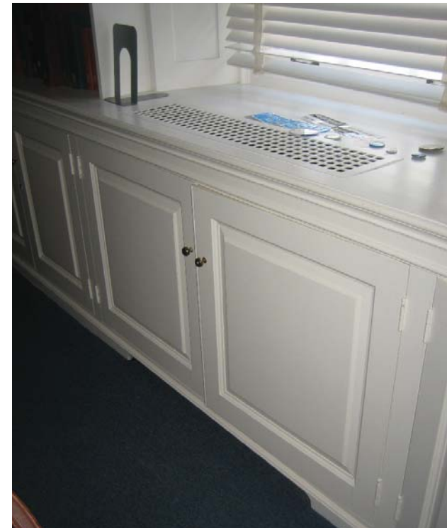
Air handling unit inside cabinetry at the Library/Parlor
