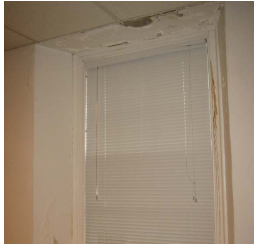
Plaster and paint damage in the Decatur Room. This is the typical of damage found in other spaces.
