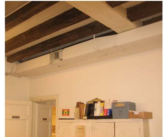
Existing wooden ceiling joists originally used in the White House. These will be highlighted in the proposed project.
