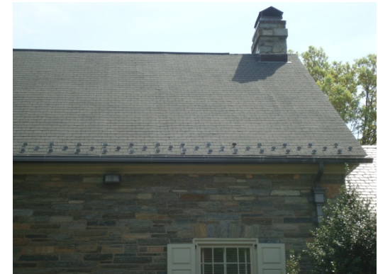
The asphalt shingles are about 20 years old and are beginning to crinkle, the first sign of age.
